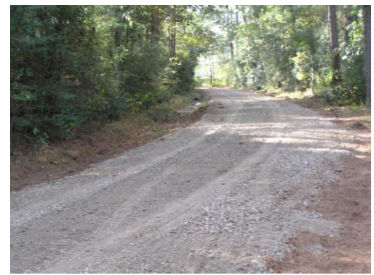
Though more expensive than planting grass, rock is an excellent choice for roads that remain wet for extended periods of time or for roads with a high erosion potential.
